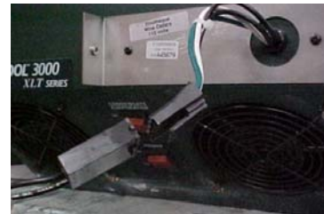
Black bypass plug connection, used on most units 2003 and beyond. On all WhisperKOOL models the bypass plug connection is located on the front of the unit, behind the thermostat.
